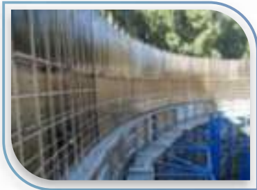
Treatment facilities, Russia.
