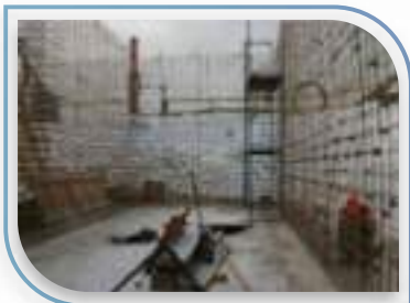
Pumping station, Russia.
